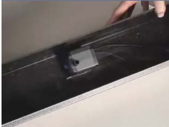
This is how the pump should rest in the tray. (Picture taken while tray is off the wall)
